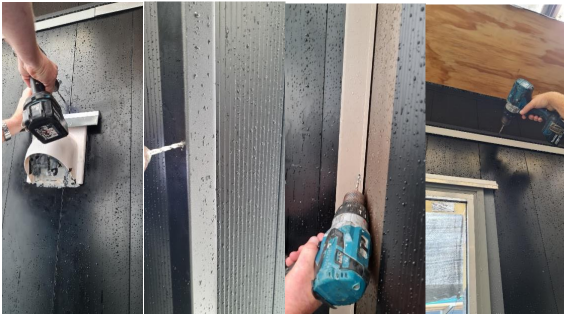
Figure 33: Holes formed for assessing cavity drainage above cowl, through corners and inter-storey joint
