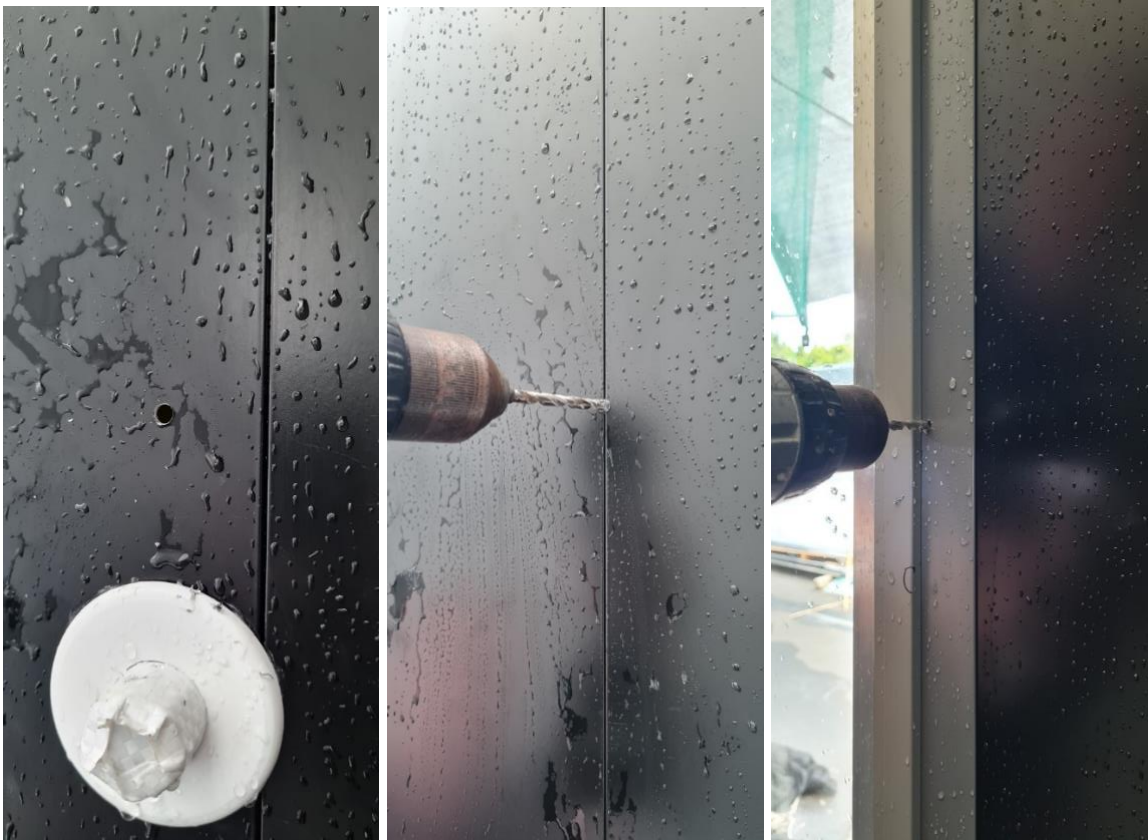
Figure 35: Holes with 6 mm drill formed above small pipe flange, through vertical joint and window jamb
