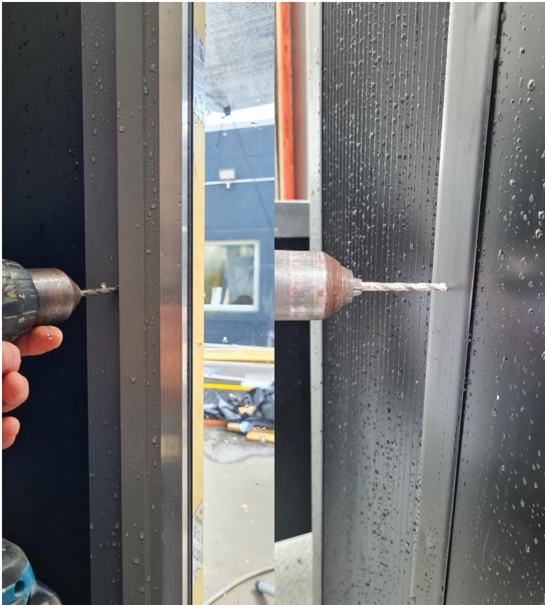
Figure 36: Holes formed through window jamb and vertical board jointer
