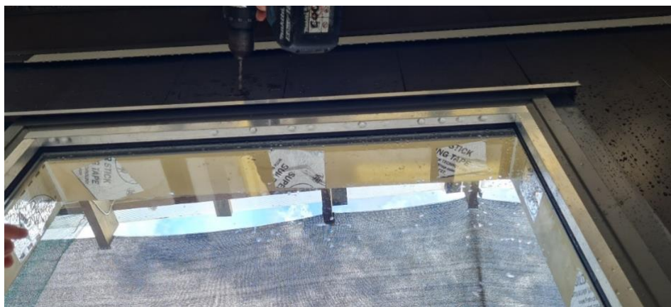
Figure 34: Hole formed about window head
