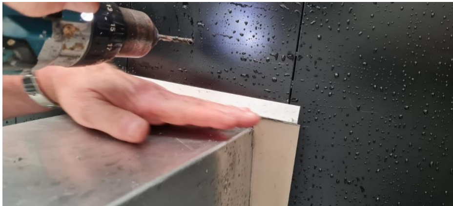
Figure 32: Hole formed above parapet saddle flashing joint
